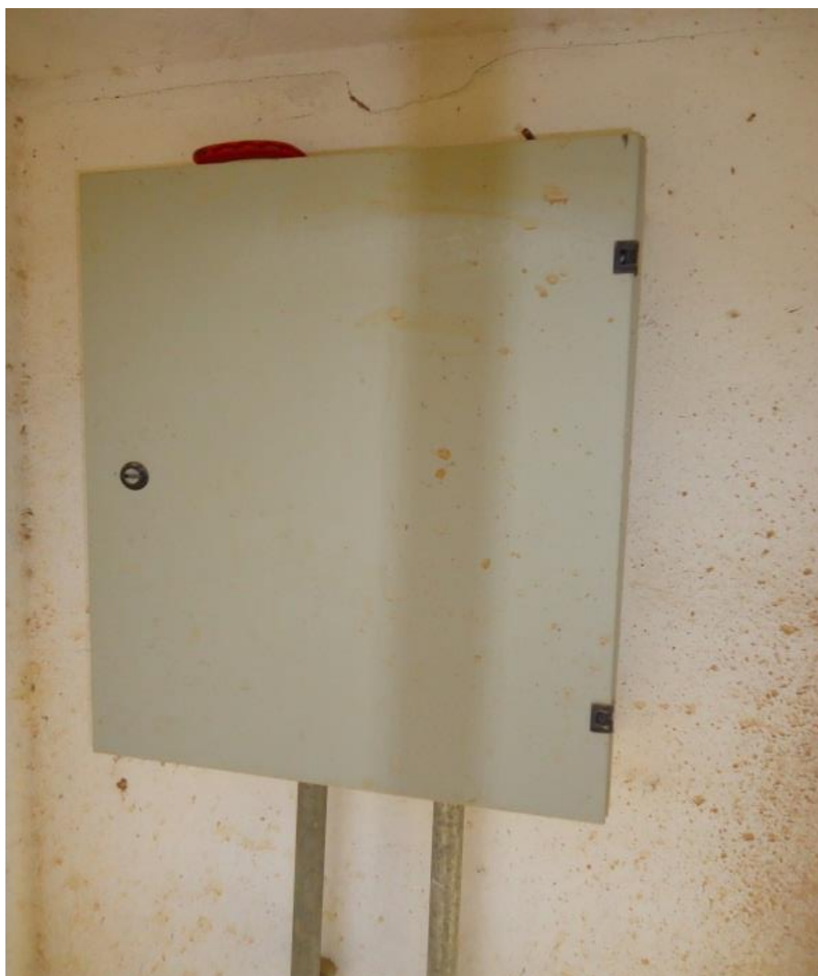
Figura 105 – Painel de Controle.
