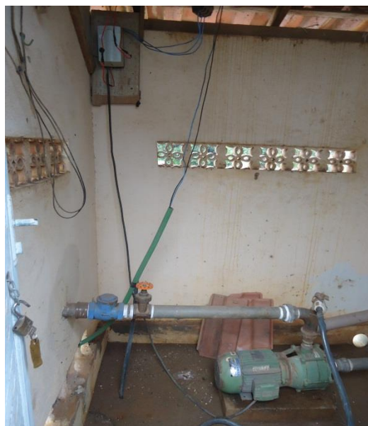
Figura 48 – Painel de Controle EEAT .
