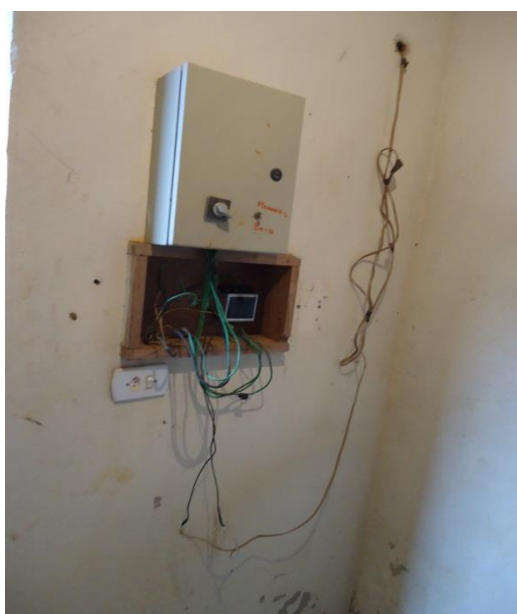
Figura 53 – Painel de Controle EEAT.
