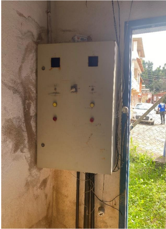
Figura 125 – Painel de Controle EEAT.
